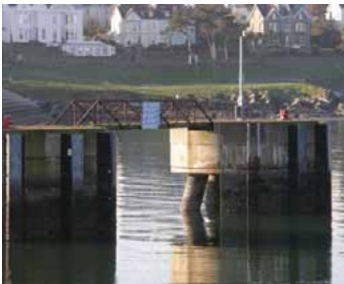
Figure 8 The Navigational Dolphins: the gap beneath the walkway has space for Black Guillemots. These gaps are quite open and spacious although a small service duct (about 12cm diameter) at the rear of the ledge provides safety from predators
